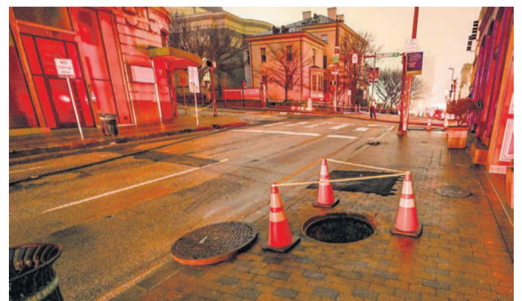
Jan. 26, 2024: An open manhole is seen on Friday, Jan. 26, 2024, along Charles Street following an underground fire late Thursday night.
